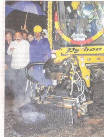
Python 5000, the advanced pothole-filling machine, at work on Race Course Road on Saturday. KPN
